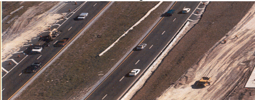
Looking East at New Eastbound I-4 at New Columbus and 50 th Street Bridges In February 2006
