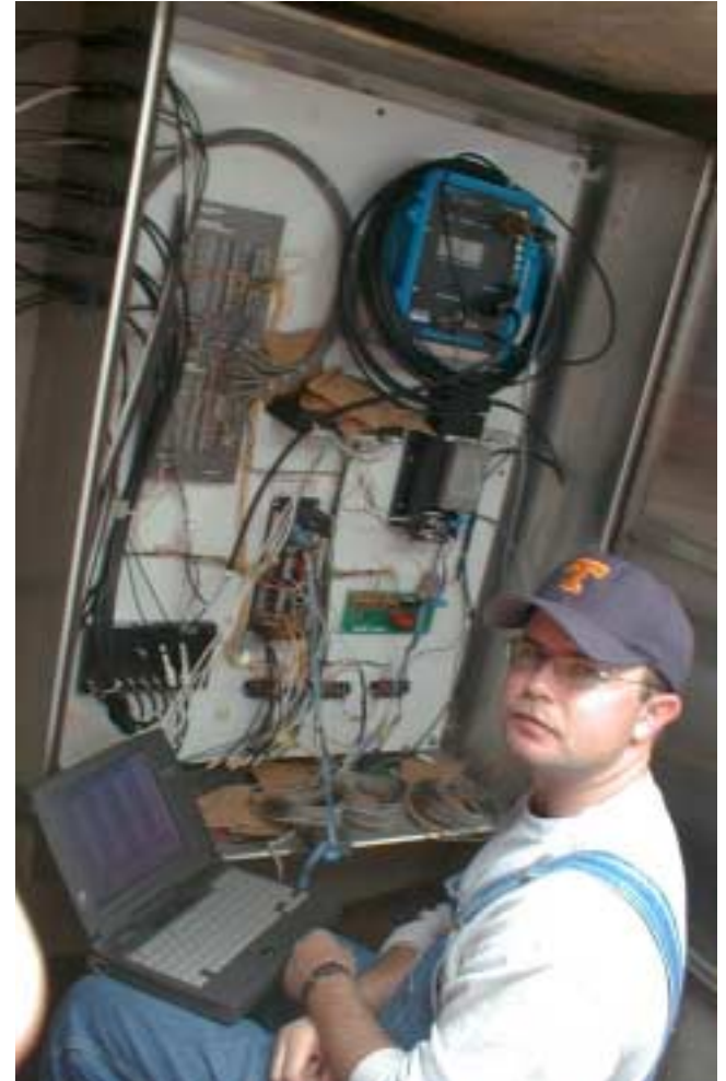
Underground Instrumentation Panel
